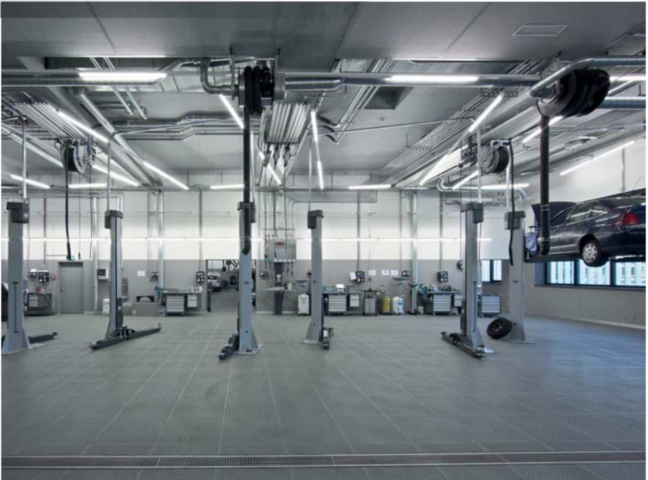
Continuous-line luminaires suspended from the ceiling illuminate the modern repair areas.
