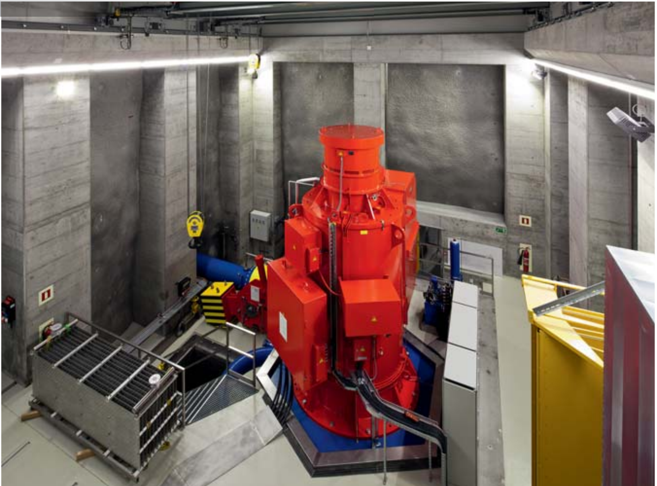
The concrete supports and foundations in the underground central station were cast in-situ. TRILUX Mirona LED luminaires ensure good illumination.
