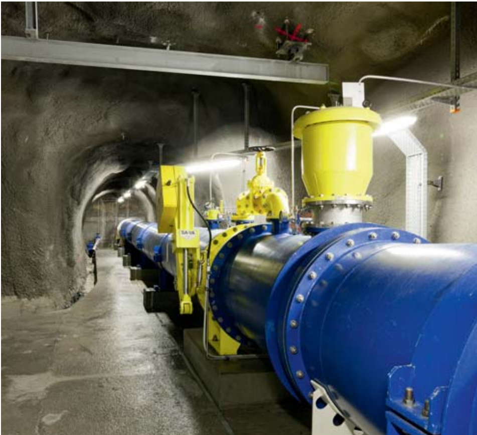
The throttle valve (marked yellow) protects the plant from overflowing in case of a defect in the pressure line.
