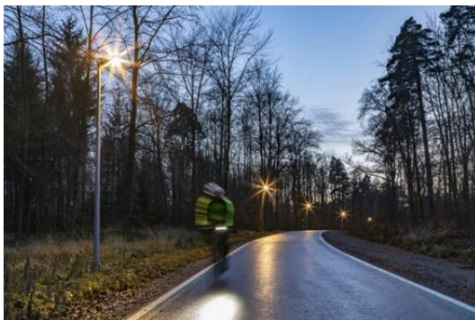
[Photo: TRILUX_Cycle Route] Very sustainable: 130 Lumega IQ 50 luminaires were networked with LiveLink Outdoor on the 8 km long cycle path from Stuttgart to Sindelfingen. An intelligent feature of the system is "tracking light".
